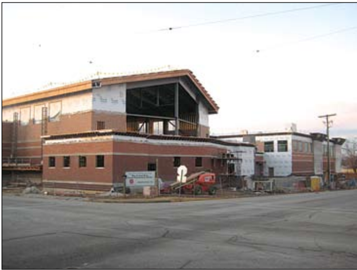
Future site of $20 million Ray and Joan Kroc Community Center located in downtown Quincy.
